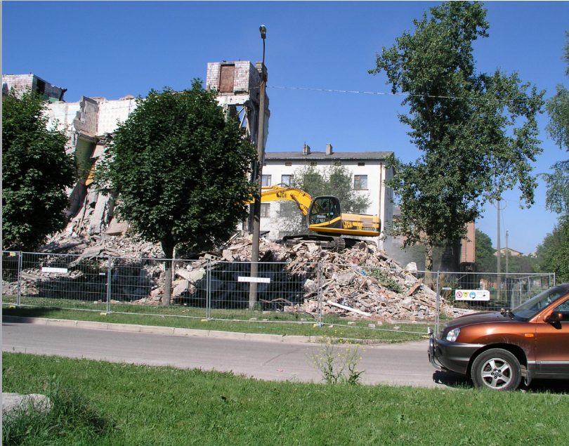
Figure 3. The demolition of a 5-story house built approximately in the 1970s on 6 th of July 2005 on the corner of Vahtra (maple; formerly Varese—not crow but a historical political figure) and Olevi (character from the national epos; formerly Comsomol) Street. Photo: Anu Printsman).
