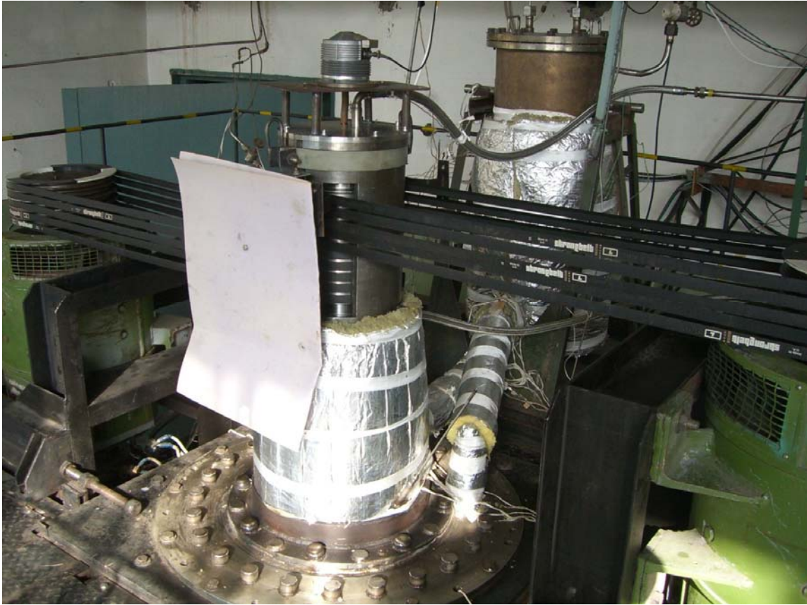
Fig. 1: The newly installed magnetic coupler, connected by 2x5 belts to the two 100 kW motors.
