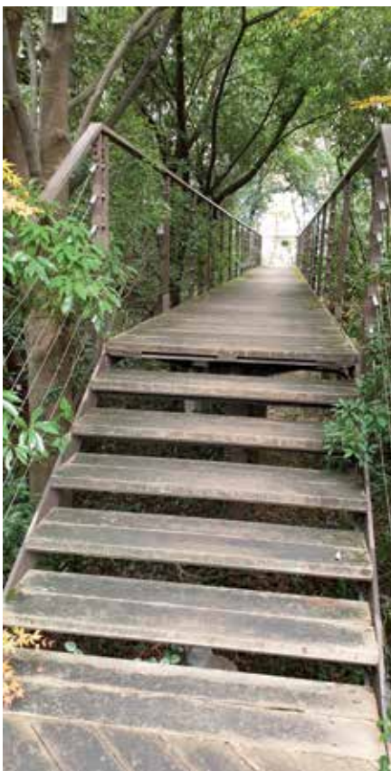
Pic. 17. A bridge leading to Inochi no Mori . Photo by A. Haijima, 2019
